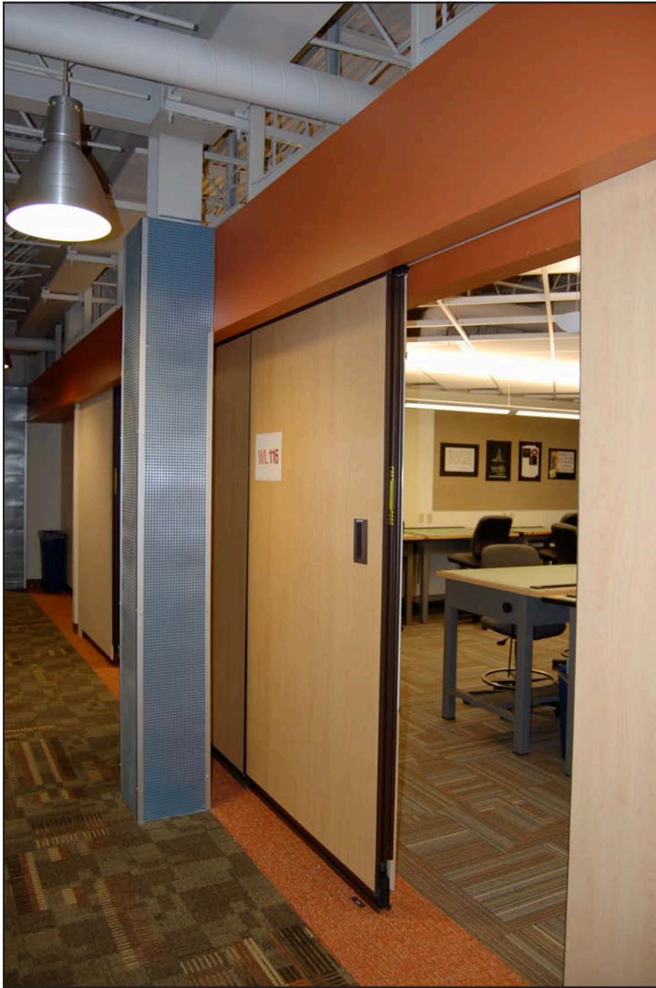
La Roche remodeled the first floor of the Wright Library for Graphic and Interior Design. © Stephanie Jones
